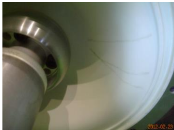
Fig. 6 Surface discharge of branch busbar with original structure
